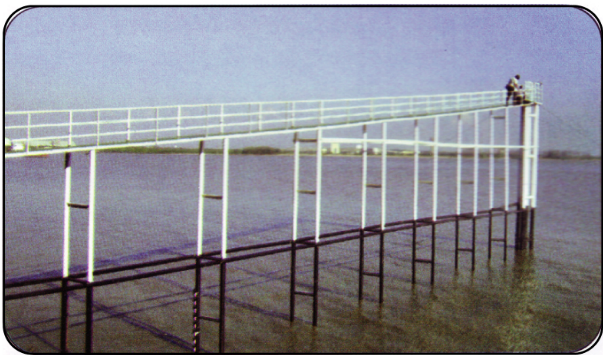
Auto Tide Gauge Station at Khal 18
